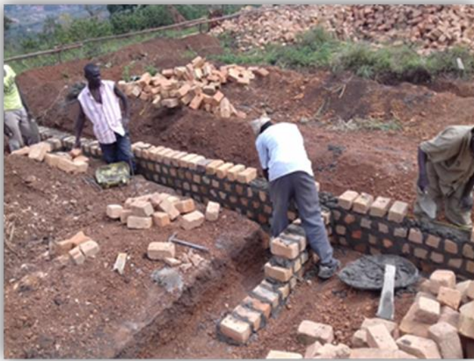
Brick laying went on for two weeks to bring up the foundation to above ground.
